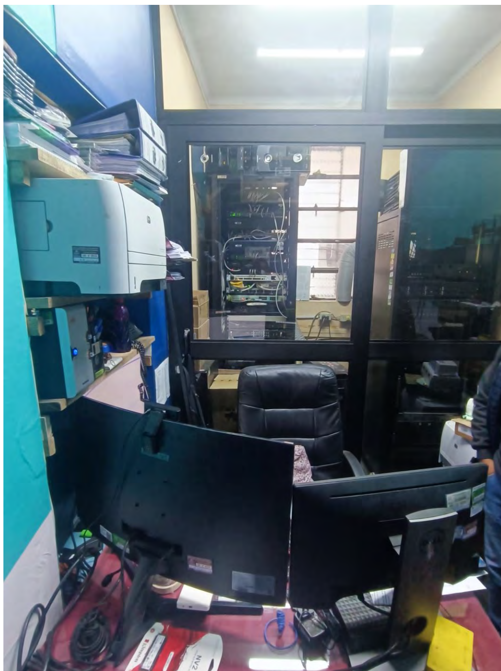
Area de TIC del hospital departamental ZCV
